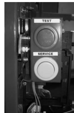
Test and Service Panel
